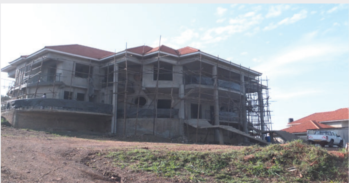
The view of the residential home in Lweza being constructed by Aswangah construction services ltd
