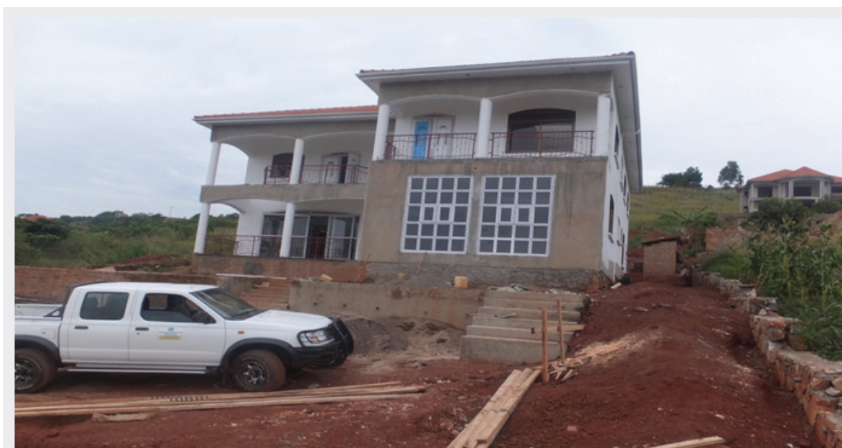
Finishing works in progress for Private developer house at Akright Kakungulu Estate
