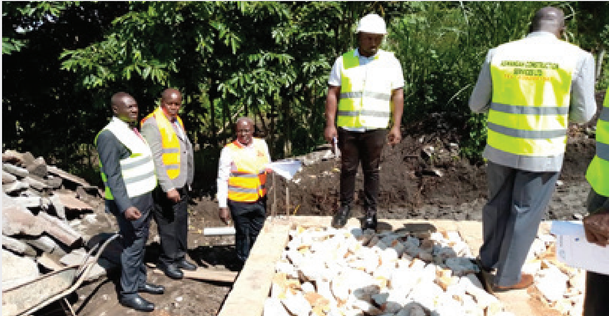
| Pre-fabricated office blocks at Mountains of the Moon University, Saaka campus – Fort Portal (in progress) |
